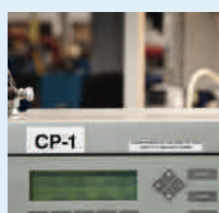
Control Panel and Electrical Panel Labels
