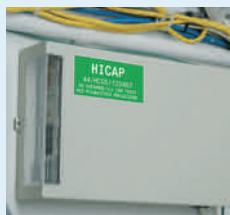
Control Panel Labelling
